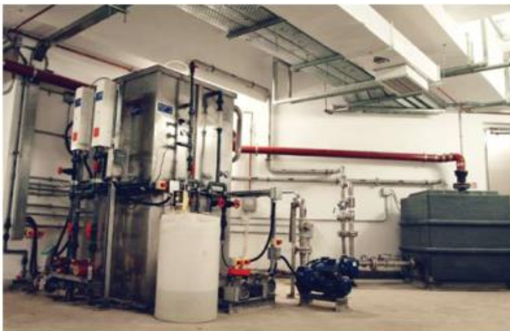
Figure 9.1 Typical appearance of a small scale MBR plant (Source: Dunwell's Bio-Toilet in Zero Carbon Building, Dunwell Group)
